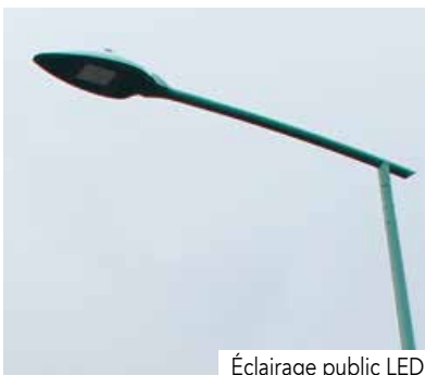
Éclairage public LED
